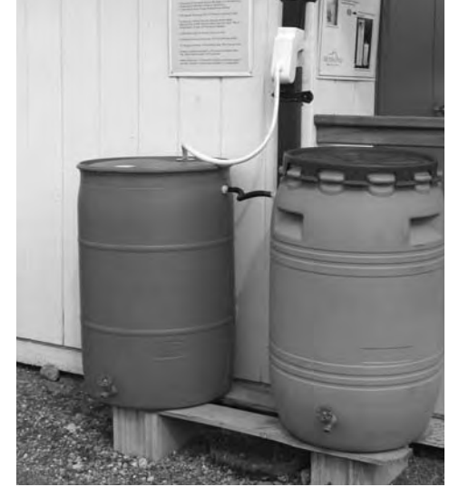
Shown are two interconnected rain barrels. An aftermarket diverter is used to divert rainwater from the existing downspout to the rain barrels where it can be stored for hand watering.
