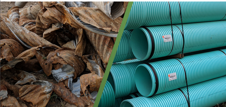
Pictured: Old vs. new storm sewer mains installed in Phase 1 construction in 2018.
